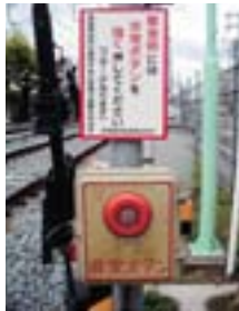
踏切支障報知装置 ▶
